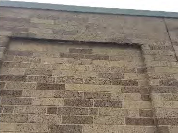
Some delaminating lintels
