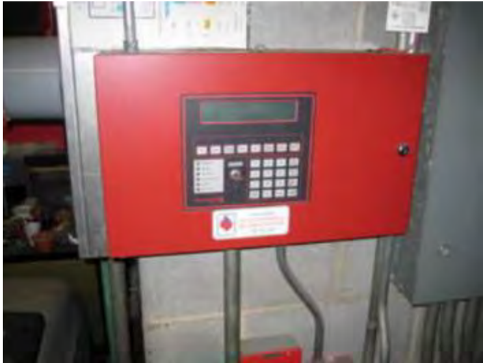
Fire alarm system is inadequately provided, doesn't meet NFPA or Ohio Building Code, nor will support a fire suppression system
