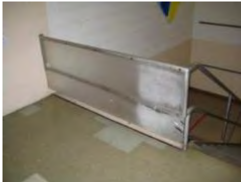
Non-Code compliant hand/guardrails
