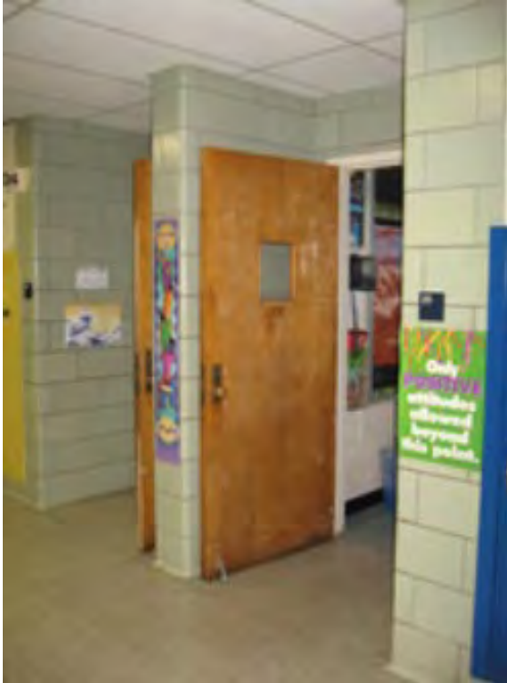
Worn doors without ADA hardware
