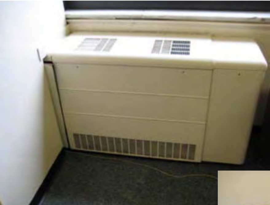
Unit Vents do not provide code levels of fresh air
