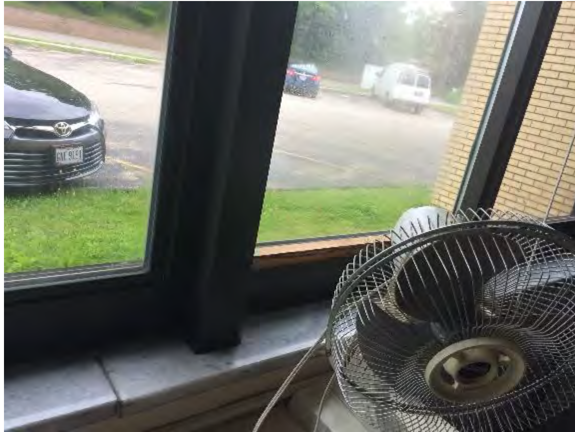
1982 windows – seals and hardware failing (note window fogging occurring)
