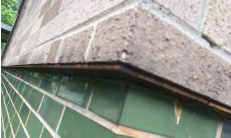
Rusting perimeter angle
