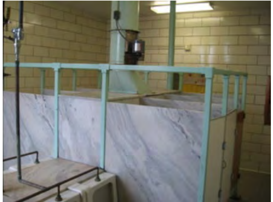
Boy's restroom in dated and worn condition and lacks ADA fixtures
